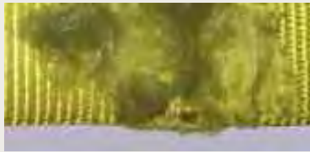
Excessive abrasive wear
